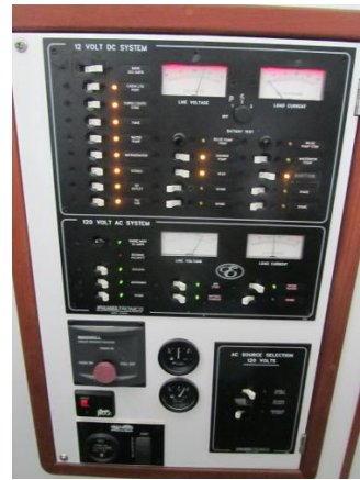
36' Endeavour electrical panel
