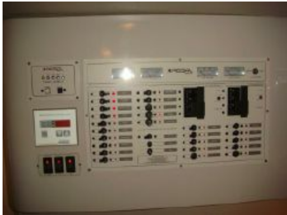
> 40' Regal electrical panel
