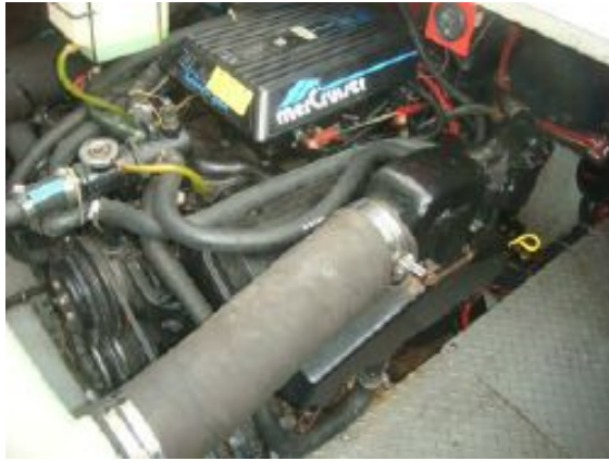
> 40' Regal port main engine
