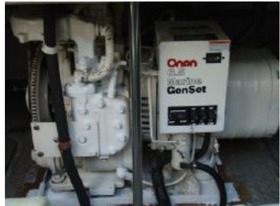
> 43' Regal generator photo1
