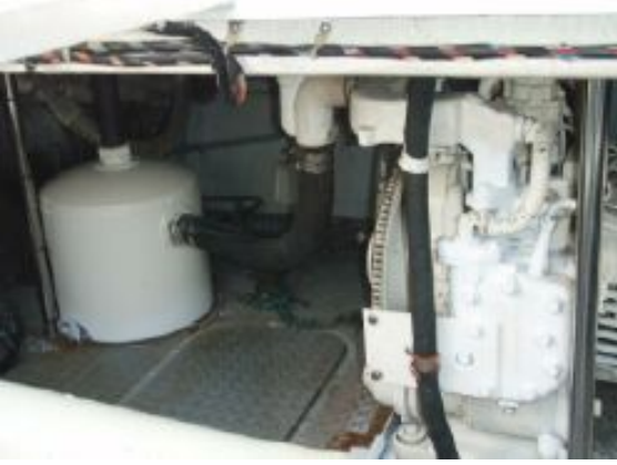
> 43' Regal generator photo2
