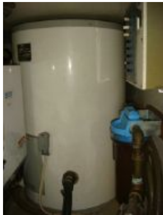
> 60' Custom Trawler water heater
