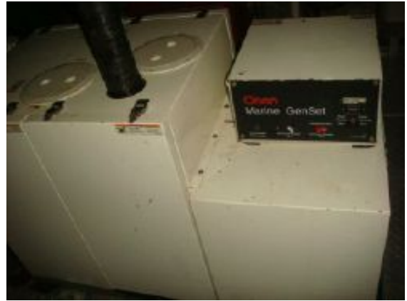
> 60' Custom Trawler generator soundbox
