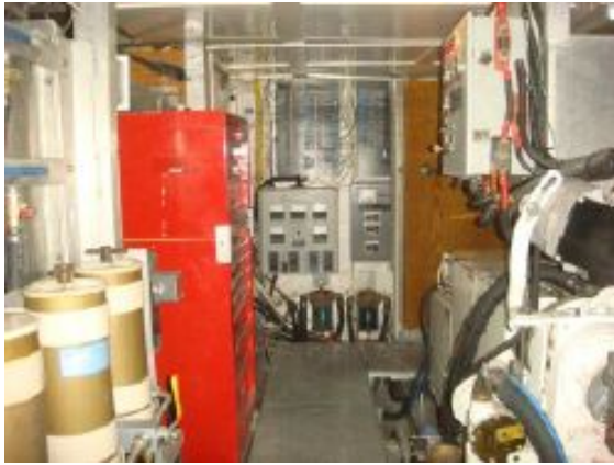
> 60' Custom Trawler engine room port forward
