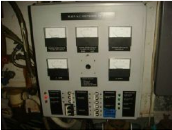
> 60' Custom Trawler engine room electrical panel
