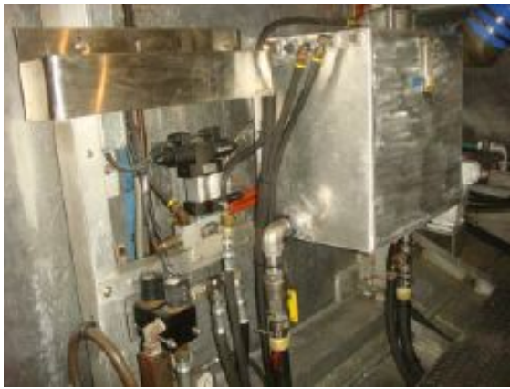
> 60' Custom Trawler hydraulic system
