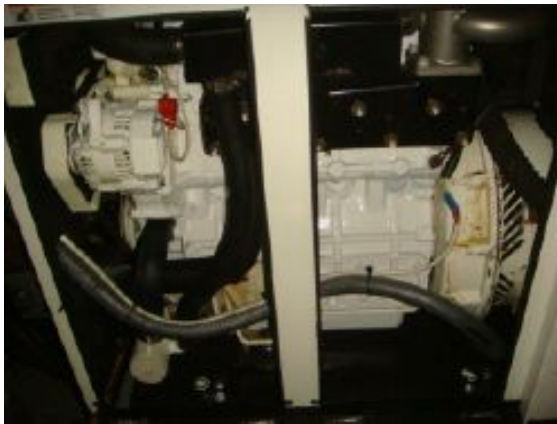
> 60' Custom Trawler generator
