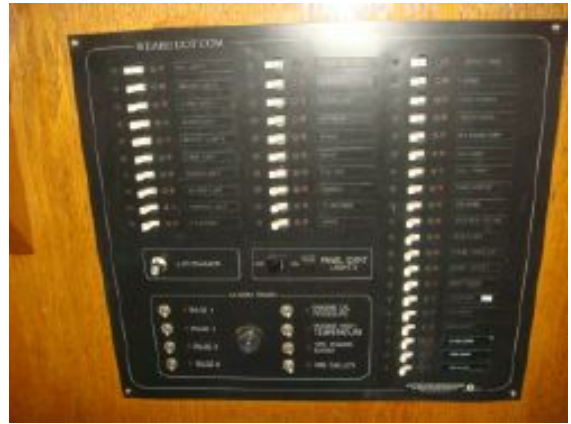
> 60' Custom Trawler pilothouse electrical panel
