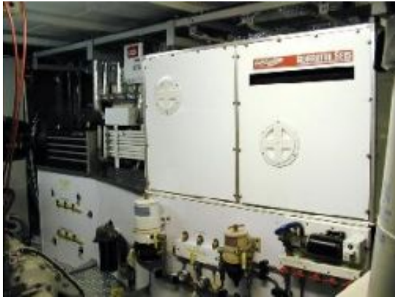
Engine Room Starboard w/ 20KW Northern Lights
