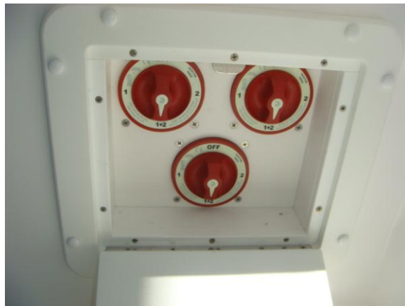
38' Renegade battery switches
