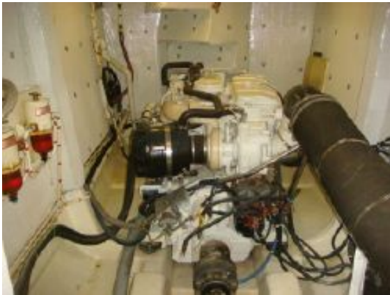
> 50' Alwoplast starboard engine room
