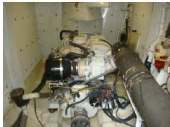
> 50' Alwoplast port engine room
