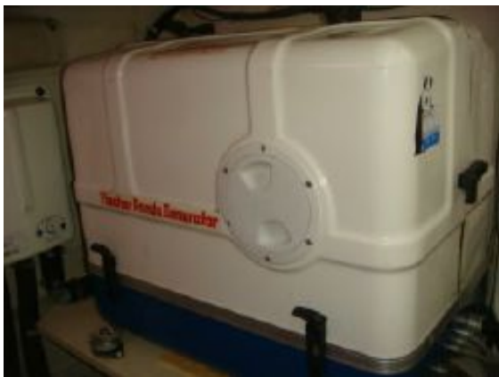
> 50' Alwoplast generator sound box
