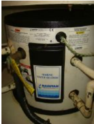
> 50' Alwoplast starboard water heater
