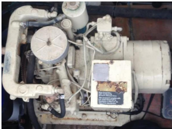
37 Silverton Sportfish Generator
