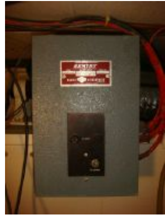
> 48' DeFever battery charger
