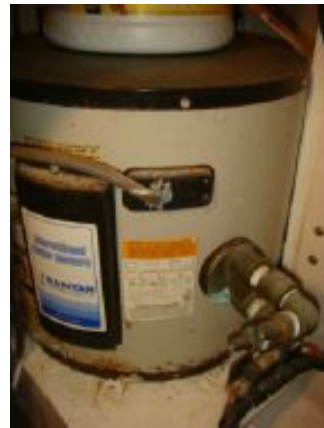
> 48' DeFever water heater
