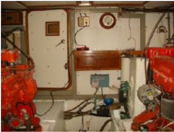
> 48' DeFever engine room forward
