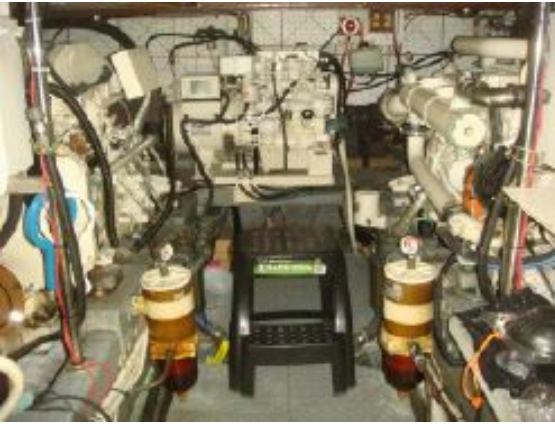
> 47' Tradewinds engine room aft
