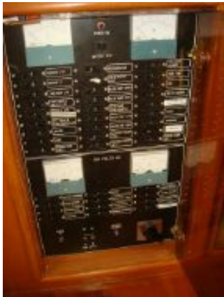
> 47' Tradewinds electrical panel
